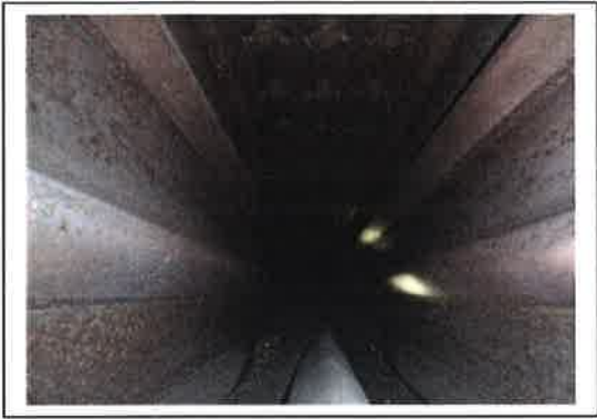
BOILER ASH @ HYDROBEAM
