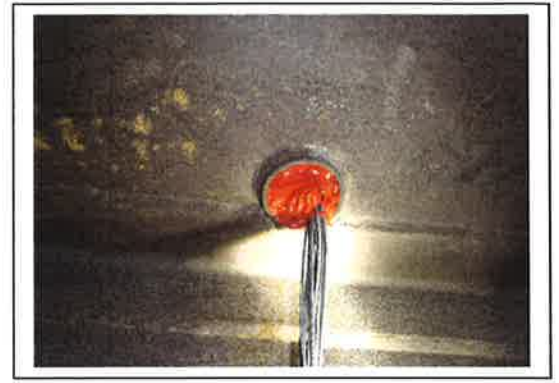
WIRES SEALED – UPPER ECONOMIZER
