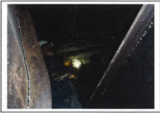
MOISTURE AT EXPANSION JOINT SCR EXITING BAG HOUSE
